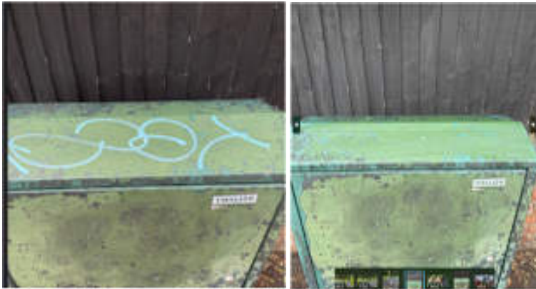
Reading Road - Cabinet outside Masonic Hall
